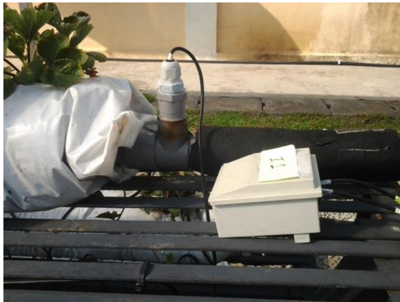
Figure 2. Temperature sensor plug into the pipe and connected to the data logger
